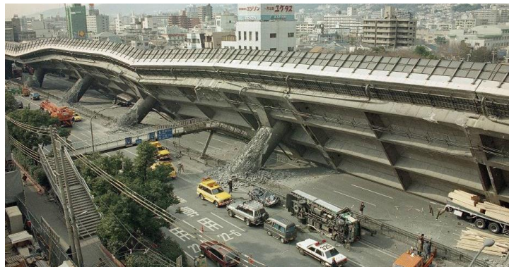
FIGURE 2. Higashi-Nada Viaduct collapse in the 1995 Hyogo-Ken Nanbu earthquake. (Source: EERI, The HyogoRen Nambu Earthquake, January 17, 1995, Preliminary Reconnaissance Report, Feb. 1995.) [4-7]
