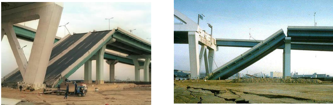
FIGURE 1. Nishinomiya-ko Bridge approach span collapse in the 1995 Hyogo-Ken Nanbu earthquake (Kobe Collection, EERC Library, University of California, Berkeley) [4-7]
