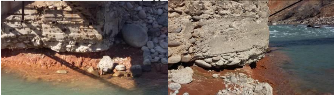
FIGURE 6. General view of the locations and conditions of bridge supports (Photo by Abirov R.)
