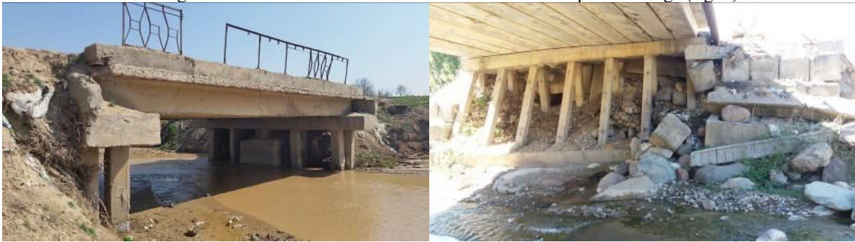
FIGURE 4. Soil subsidence due to insufficient compaction and soil washout from under transition slabs (Photo by Abirov R.)
