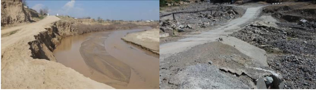
FIGURE 3. Washed out roads (Photo by Abirov R.)
