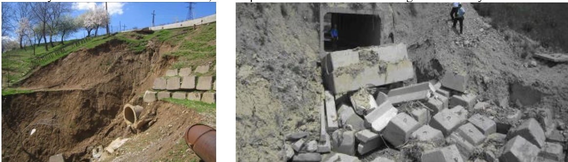
FIGURE 2. Road sections damaged due to loss of foundation bearing capacity, Uzbekistan (Photo by Abirov R.)
